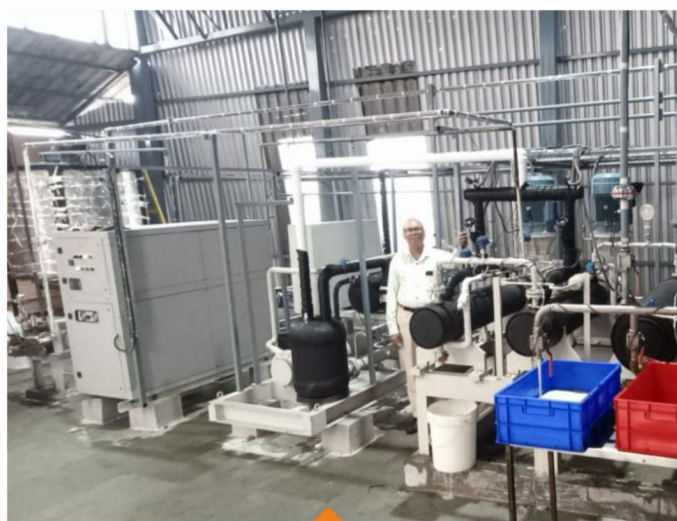
REFRIGERATION UNIT INSTALLATION IN A BUTTER MANUFACTURING PLANT
