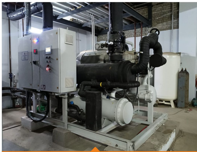
BRINE CHILLER INSTALLATION IN A PHARMACEUTICAL PLANT
