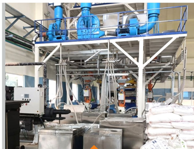
SCREW CHILLER INSTALLATION AT A PLASTIC BLOWN FILM PLANT
